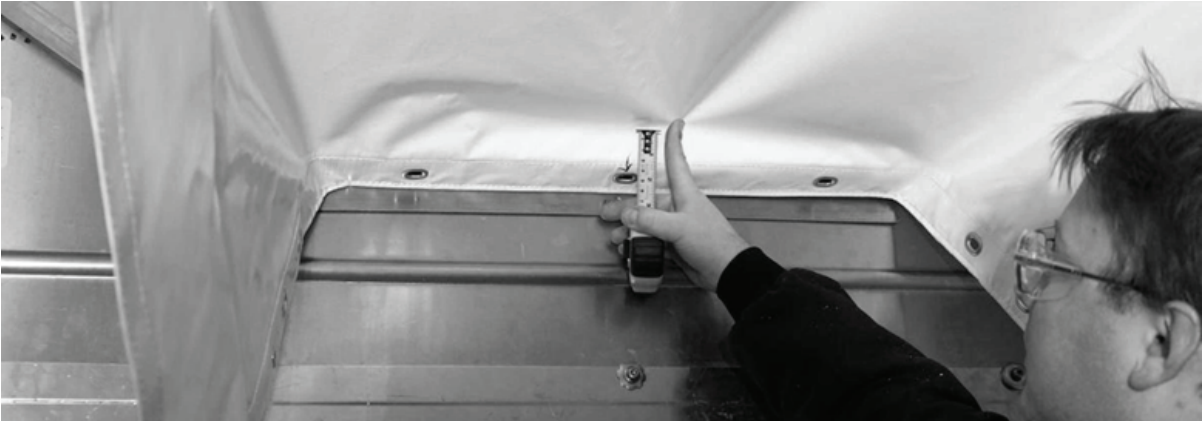
Figure 2. Chute slack in front of air outlet should be 1.00 in. to 2.00 in.
